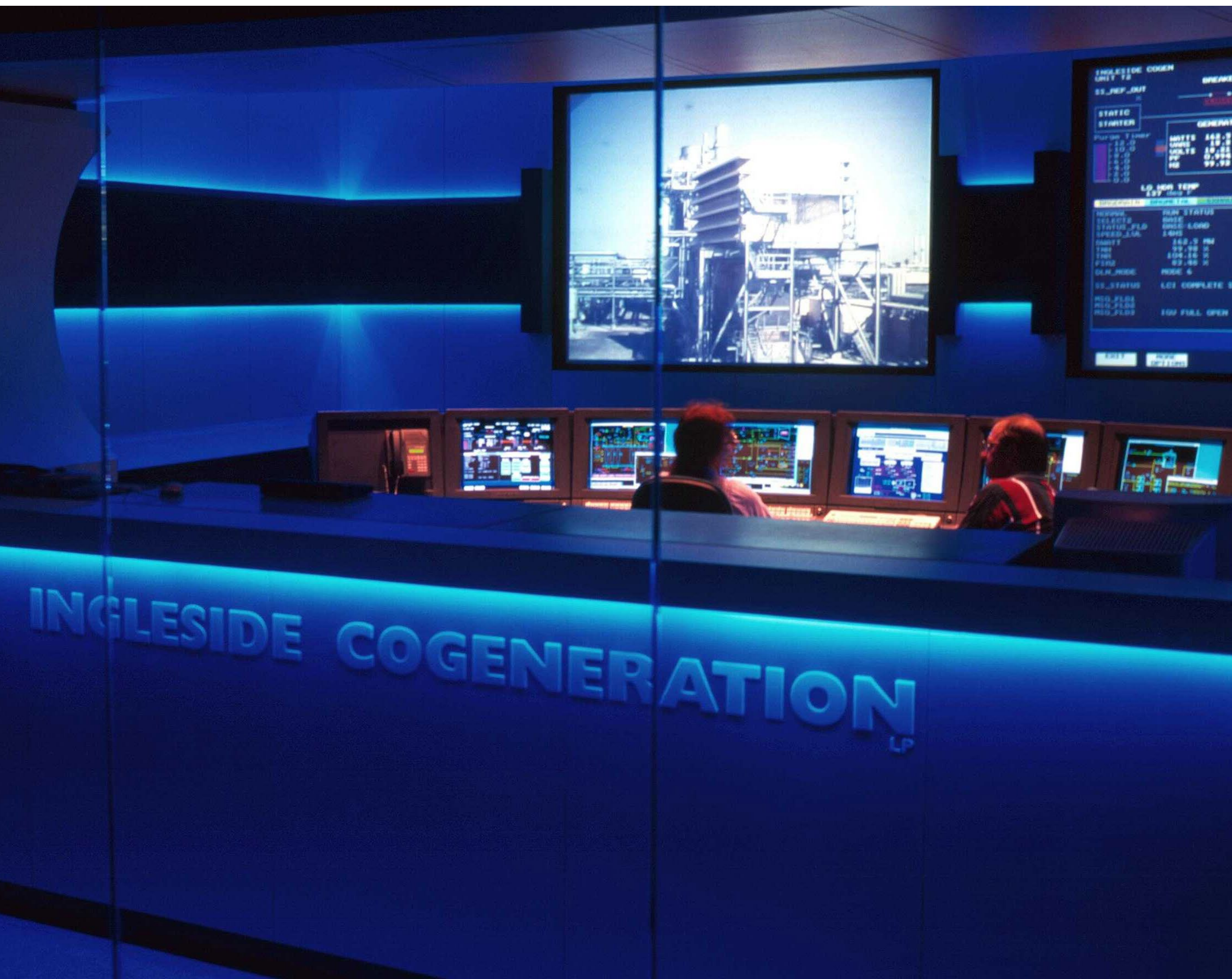
INGLESIDE COGENERATION CONTROL ROOM, INGLESIDE, TEXAS
