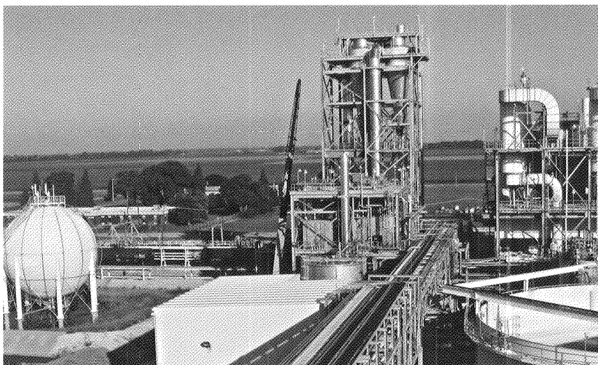
Georgia Gulf PVC Modernization Project Plaquemine, Louisiana
