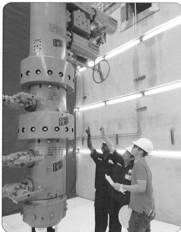
Designed-for-purpose platform wellhead system
