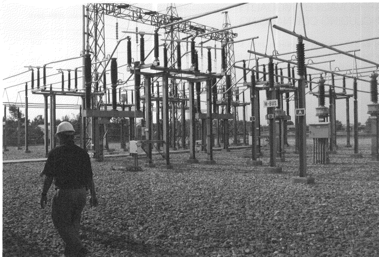
This Cambodia Power Transmission Lines (CPTL) Project benefited from a $7 million private sector loan
