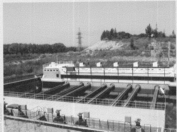
This pump station supplies precious water for rural poor
