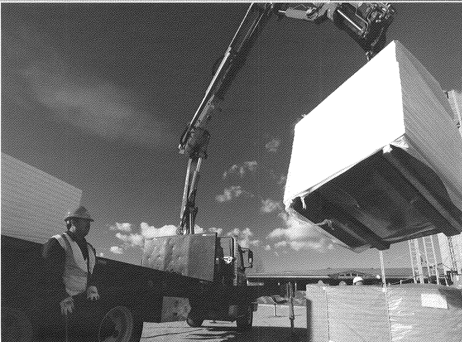
Below: Ricardo Alvaros of Allied Building Products, Denver, Colorado, operates the knuckleboom to unload commercial insulation on a new school construction job site in Boulder, Colorado. With speciality equipment such as this, Allied Building Products has the capability to deliver material directly to roofs up to 12 storeys high.
