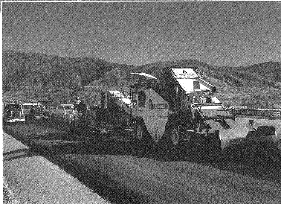
Below: Staker Parson in Utah supplied 4 million tonnes of product including road base, rock and backfill, in addition to completing all of the asphalt paving for the Legacy Parkway upgrade, a 4-lane divided highway providing congestion relief for South Davis County commuters. The project took place over an 18-month period and was completed ahead of schedule, achieving all time-related incentives available.
