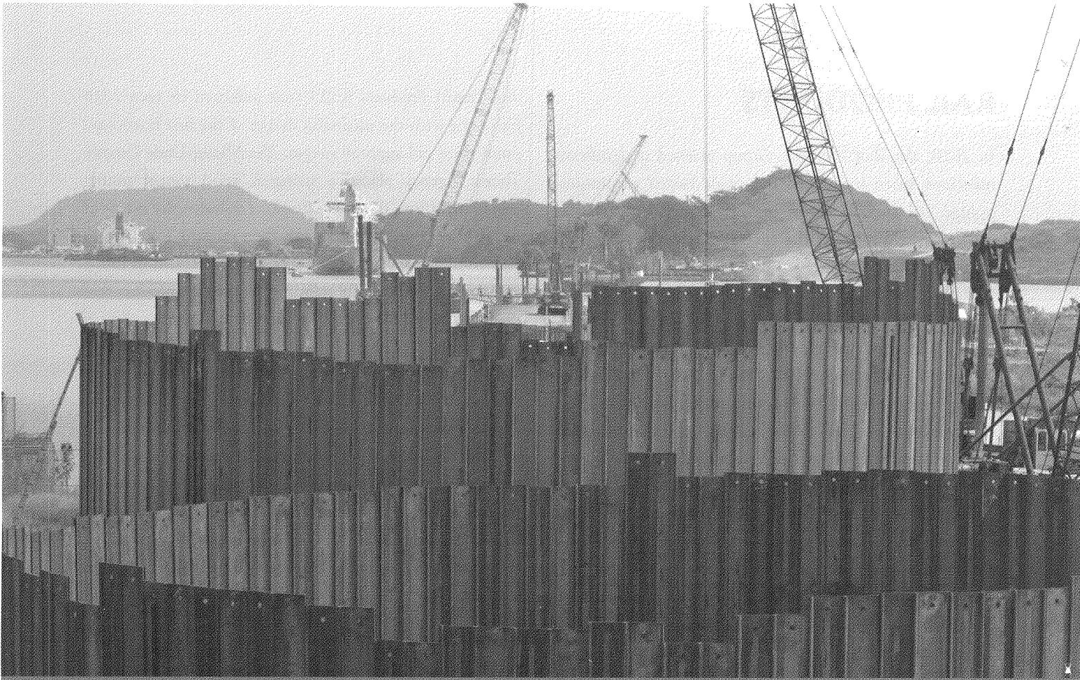
▲ L.B. FOSTER SUPPLIED PZC AND PS SHEET PILING FOR PANAMA CANAL EXPANSION COFFERDAM
