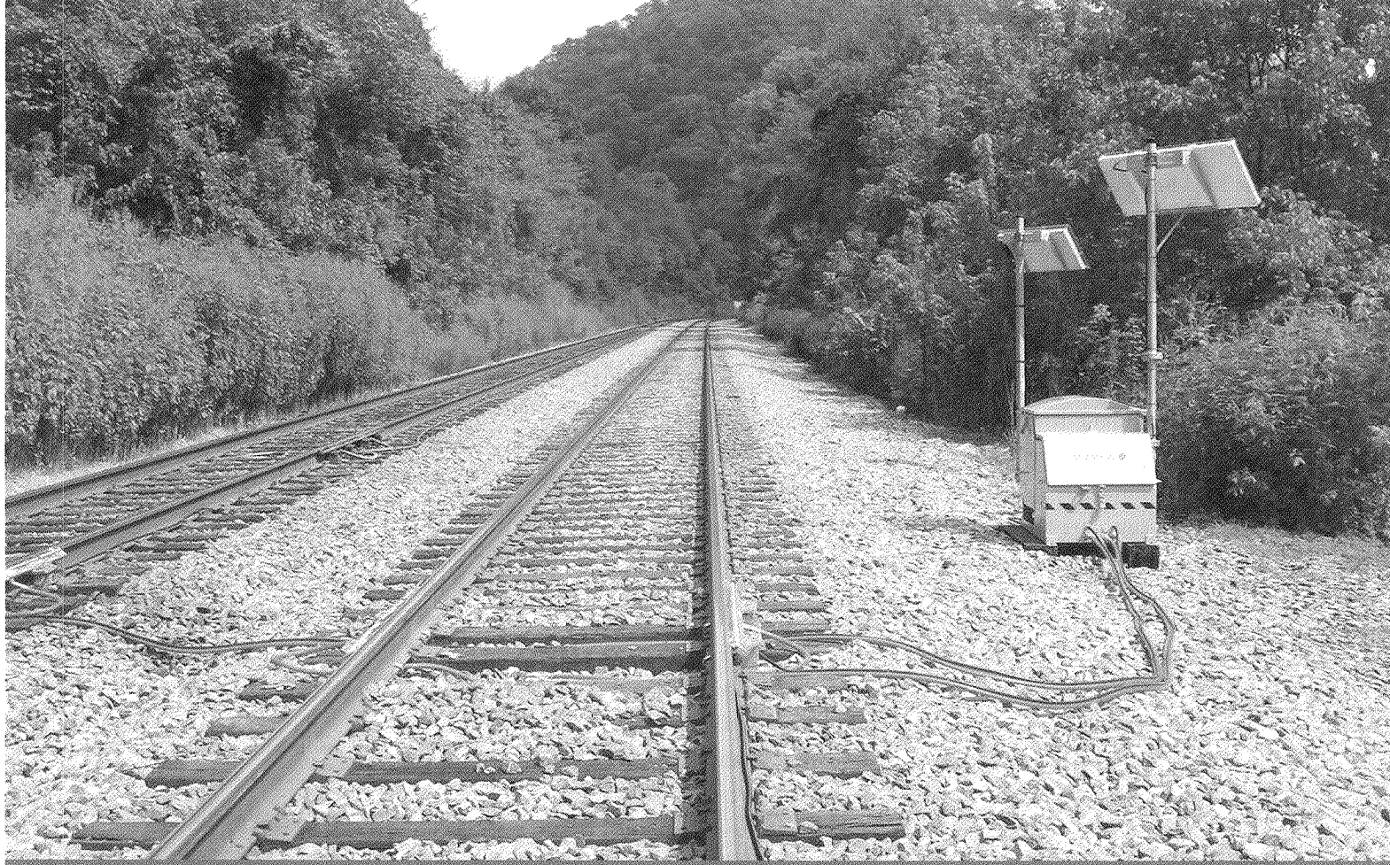
▲ WAYSIDE FRICTION MANAGEMENT SYSTEM INSTALLATION
