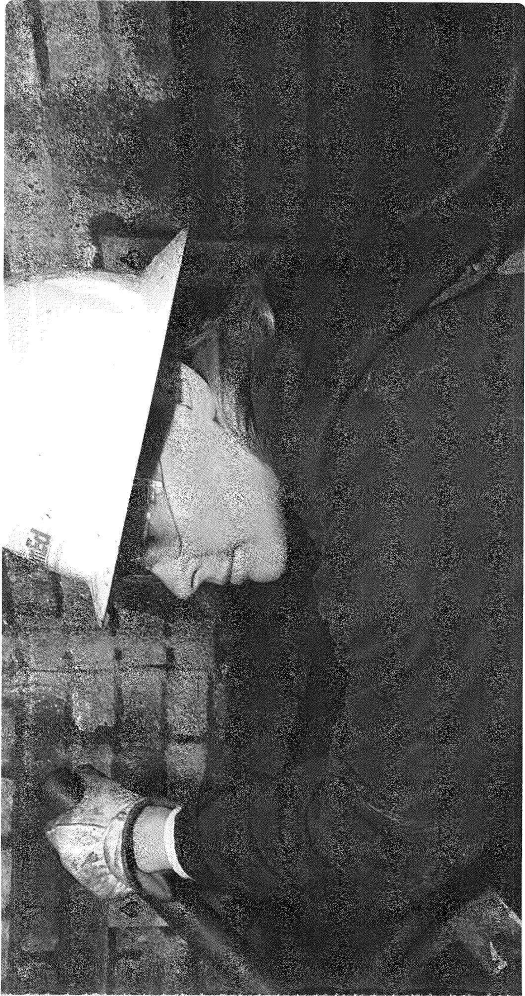
In helicopters and bucket trucks, at power plants and warehouses, at substations and in commercial locations, employees like this ComEd underground cable splicer perform tasks requiring skill, collaboration, excellence and a commitment to safety.
