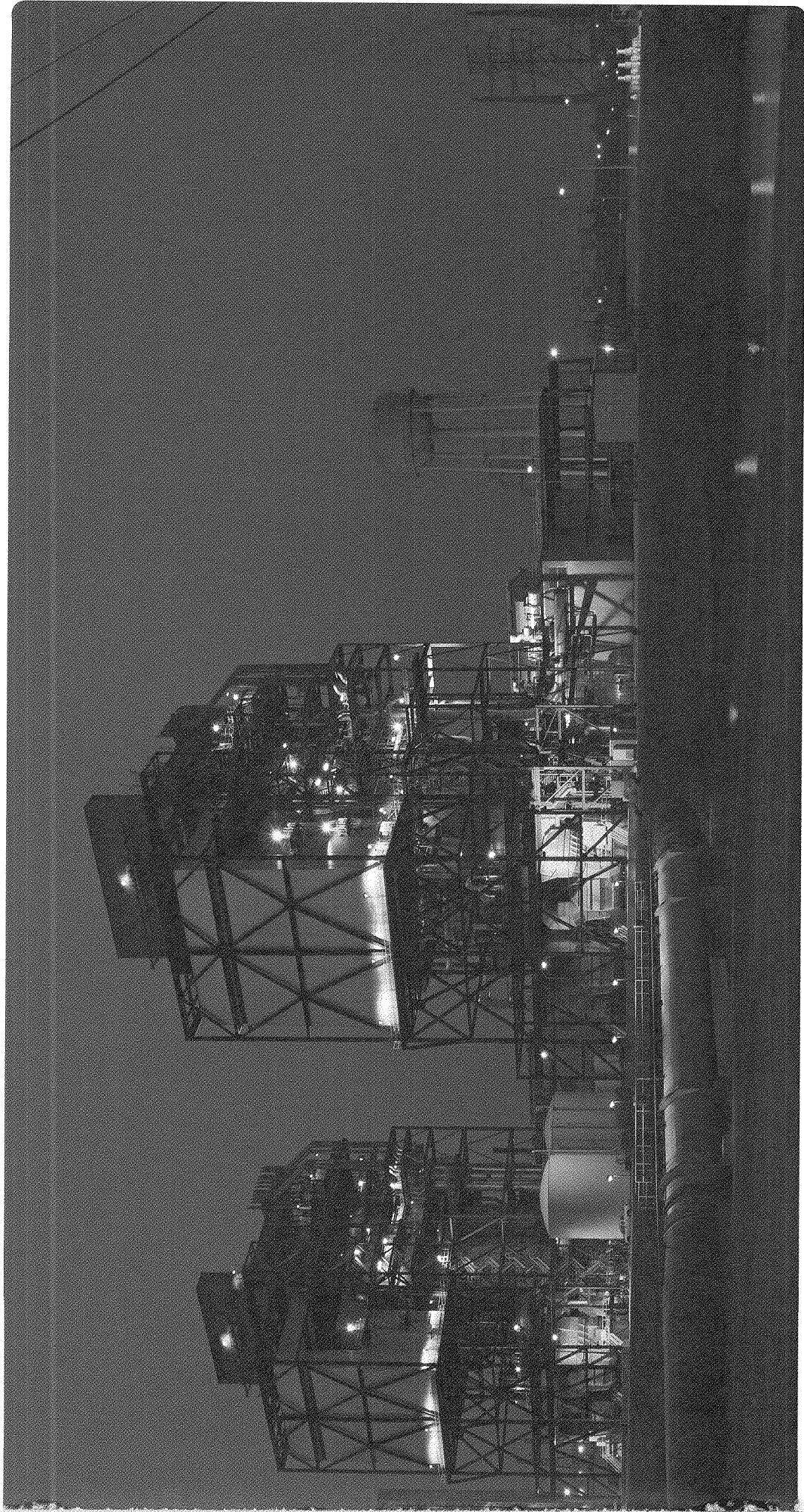
Exelon Power's Handley Station is a natural gas-burning generating facility in Ft. Worth, Texas, with three units capable of generating 1,265 megawatts when needed. New natural gas discoveries promise a more abundant supply of this critical low-carbon fuel. The cheapest way to meet new demand for electricity – when that demand materializes – is currently natural gas combined-cycle units.
