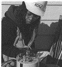
A QTI worker installs new smart meters as part of our SmartGrid Demonstration Project. The meters will provide customers with more information about their electric use.
