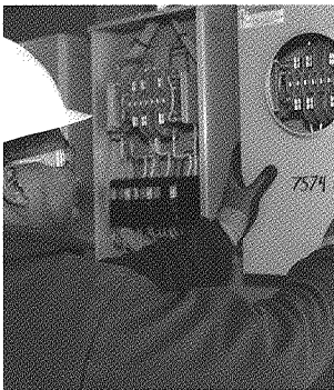
A KCP&L employee works on upgrades to the substation in midtown Kansas City, which is part of the SmartGrid Demonstration Project.
