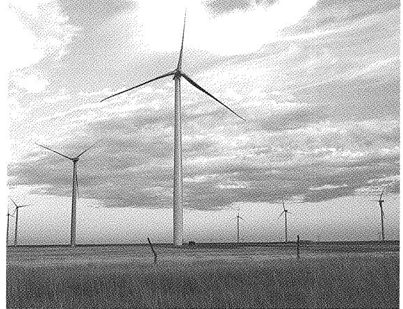
Our Spearville 2 Wind Energy Facility provides an additional 48 megawatts of wind capacity to our generation assets.
