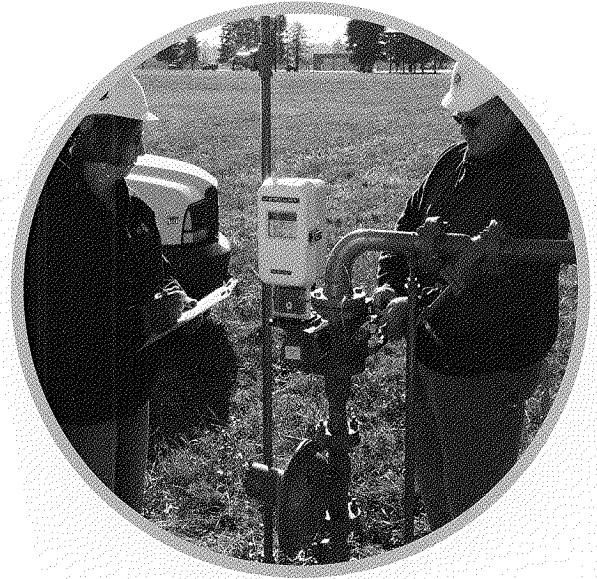
An opportunity to expand the gas operation came this year. We extended service to 56 facilities at Camp Clark, Nevada, Missouri. Camp Clark is a Missouri Army National Guard Training Site. Deanna and Ron, Gas Operations.
