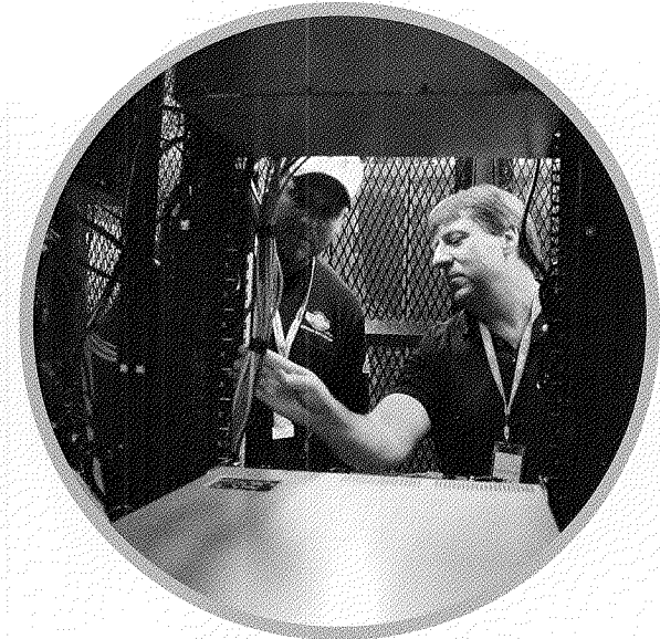
During this past year, work continued on our information technology disaster recovery site at The Mountain Complex in Branson, Missouri. All mission critical data is housed there to allow continuation of essential operations within a few hours should a disaster render the Joplin facility unworkable. Helping to make this possible are the diverse fiber optic paths provided to the complex by Empire's Fiber subsidiary. Aaron, Fiber, and Ivan, Information Technology.
