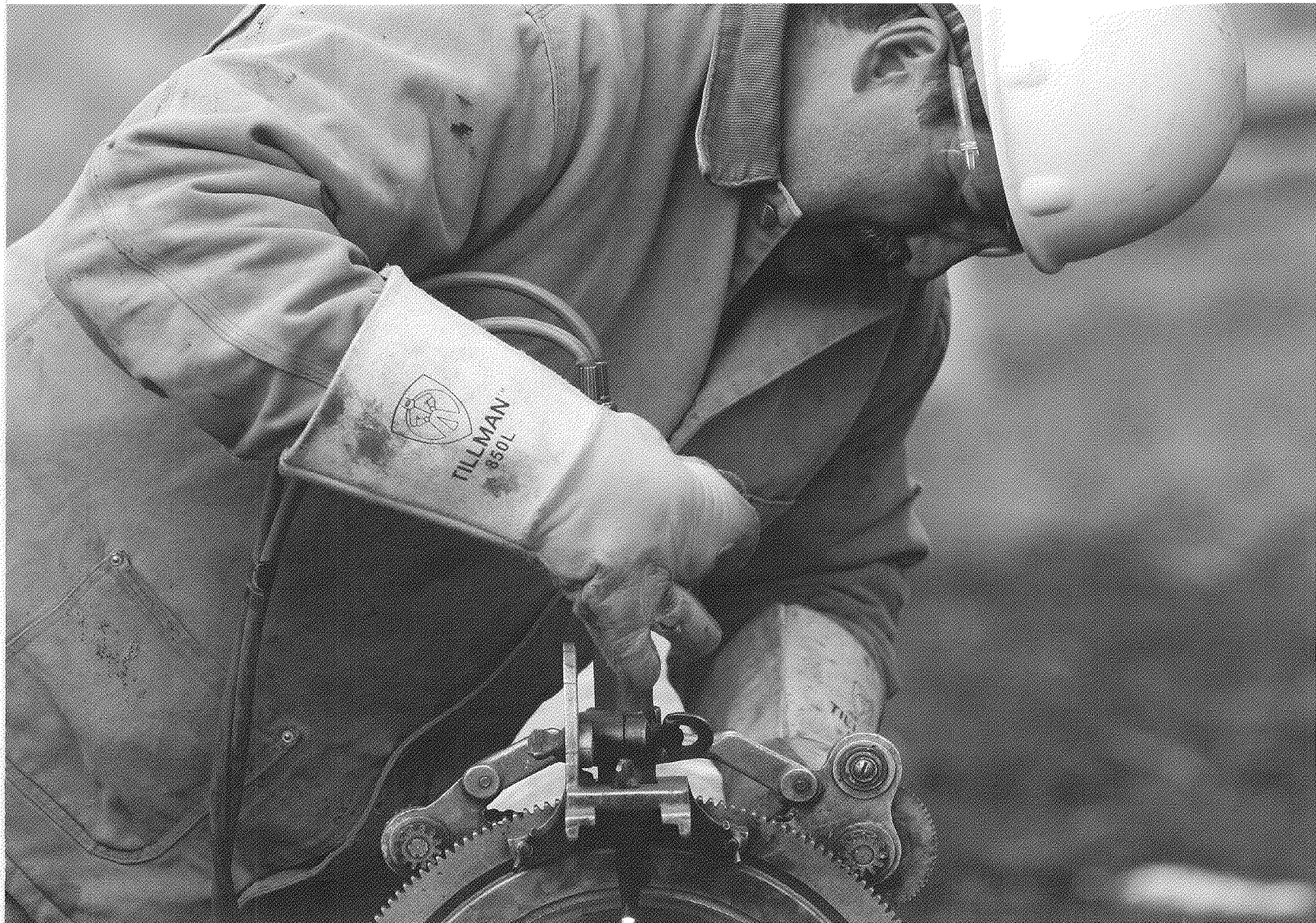
Brent Doucett of the company's Westline crew works on a steel natural gas transmission pipeline near Missoula, Montana.
