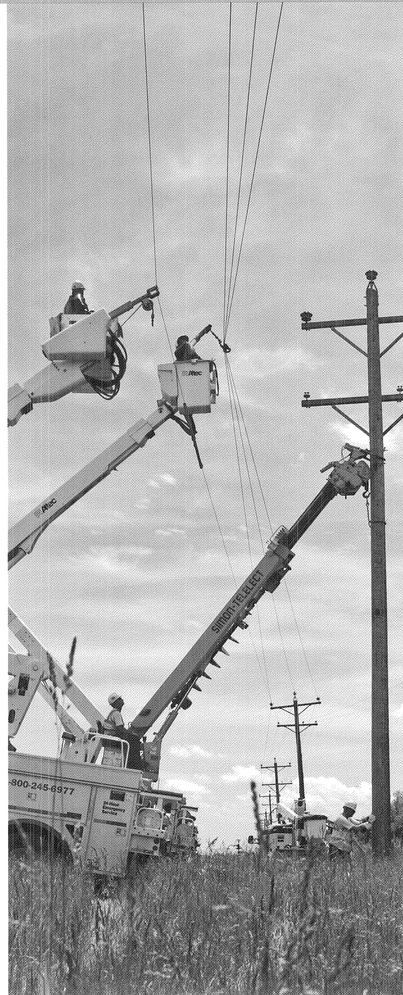
South Dakota electric crews work on a pole replacement project near Redfield, South Dakota.
