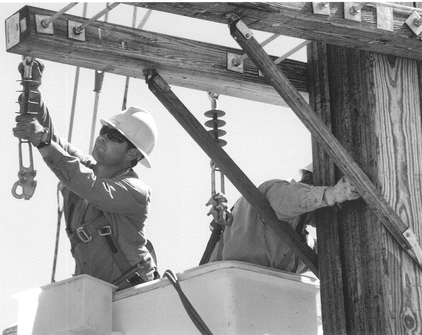
Rustin Schone and Mike McClurg work on a new feeder south of Aberdeen, South Dakota.
