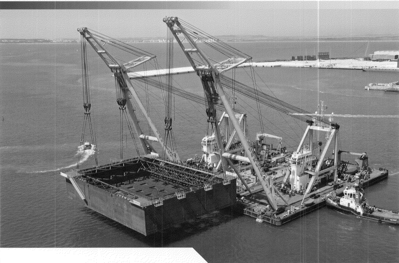
SMIT Heavy Lift installed the caissons for a new bridge in Cadiz.
