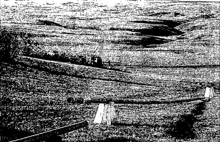
Construction crews install a four-inch plastic pipeline which will transport raw gas from two of Seneca's gas wells in the Watts field (located approximately 75 miles northeast of Calgary). The new pipeline will transport the gas to Seneca's compressor site at Watts.
