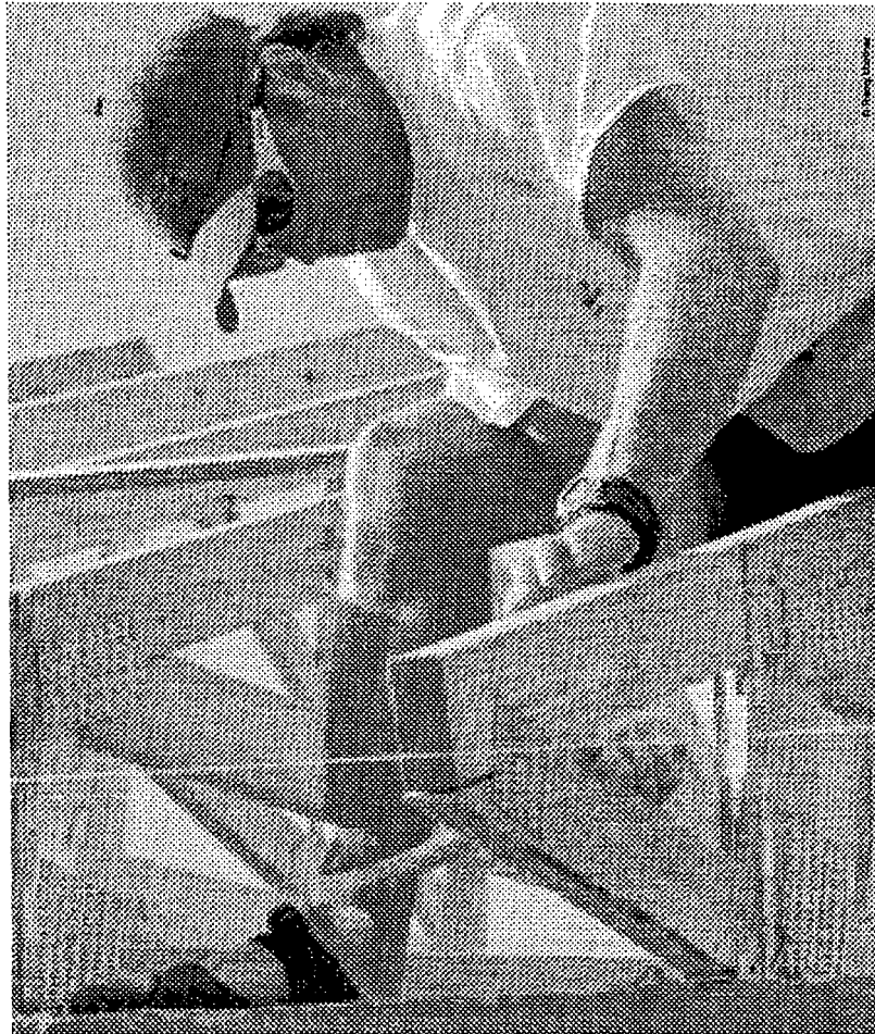
Employees gathered in Miami for the Volvo Ocean Race joined forces with the boat crew to build houses for a charitable project.
