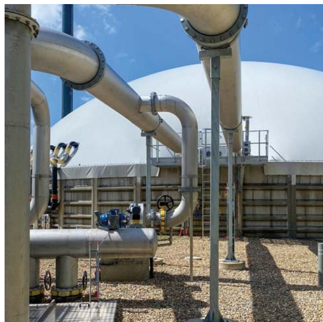
Gas process and storage equipment at the Nature Energy Korskro Biomethane Plant in Denmark.
