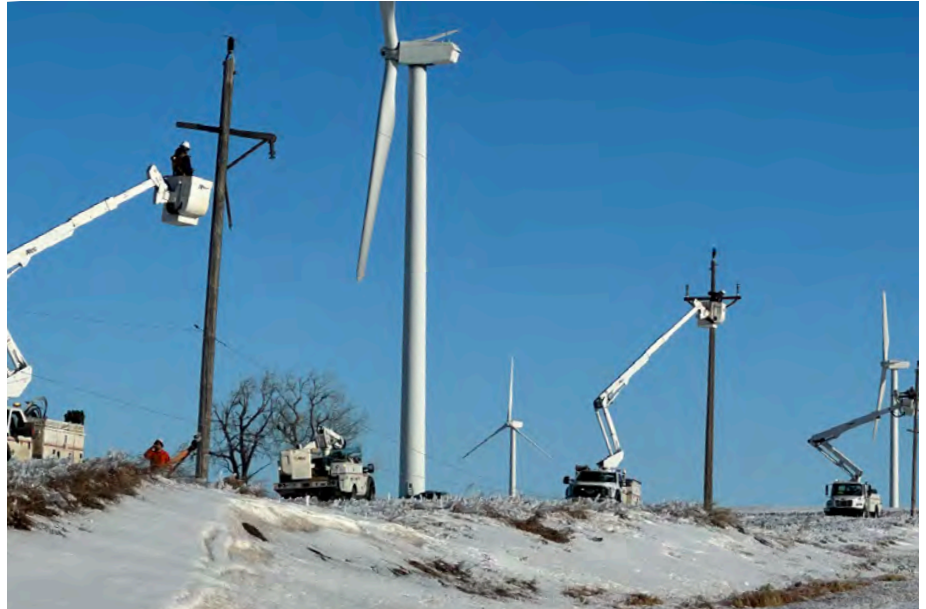
► Montana-Dakota Utilities line workers repair downed transmission lines after a December 2023 ice storm.
