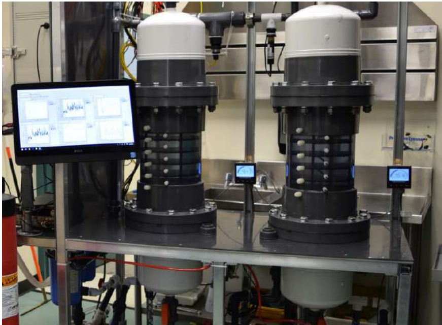
This photo shows an active AOS.
