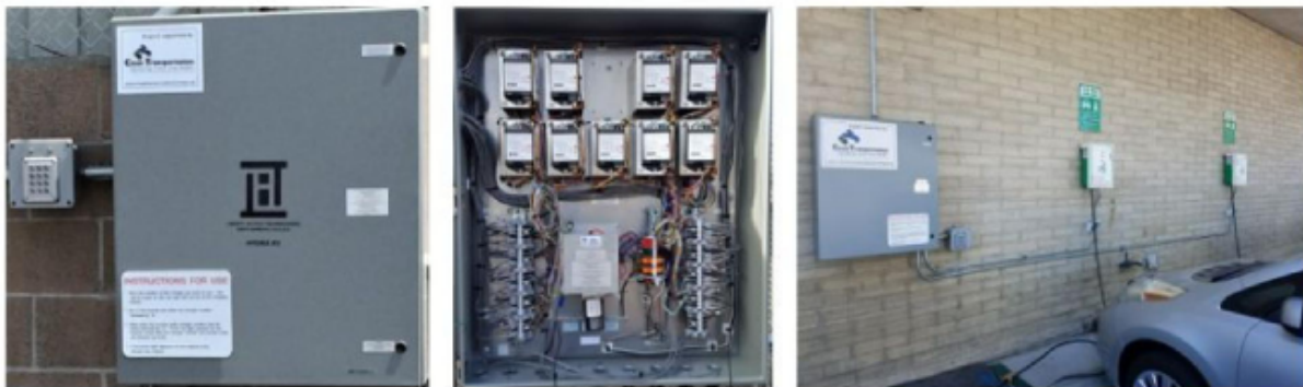
HYDRA-R Controller, Code Keypad and EV Chargers
