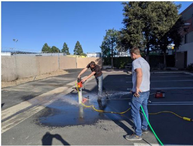
Drilling fence post holes in the parking lot with a water-cooled concrete cutting hole saw.
