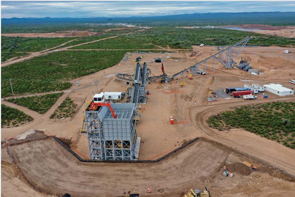
Figure 1: Crusher and Conveying Circuit
