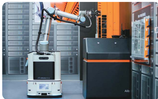
▲ Alibaba Cloud's inspection robot Tianxun is equipped with controllable arm to increase the maintenance efficiency of data centers.
