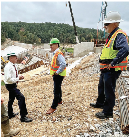
Congressman Lloyd Smucker tours Lake Williams Dam, the largest infrastructure project in York County.
