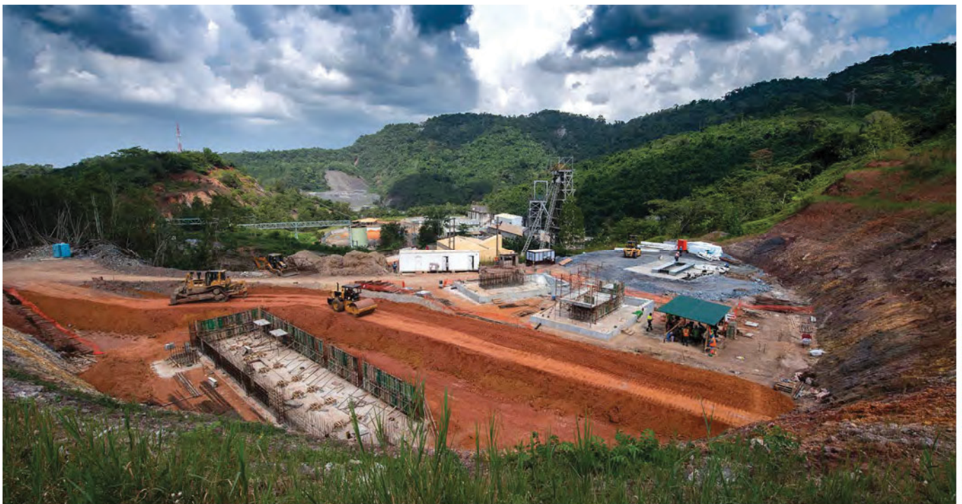
George Cappendell Ventilation Shaft fan station
