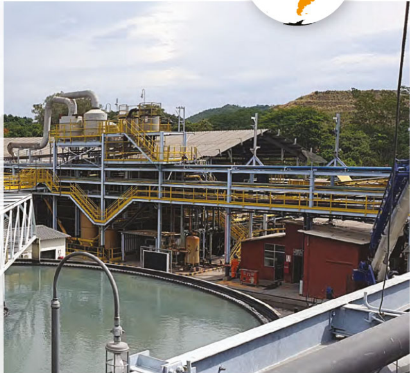
View of the thickeners at Serra Grande
