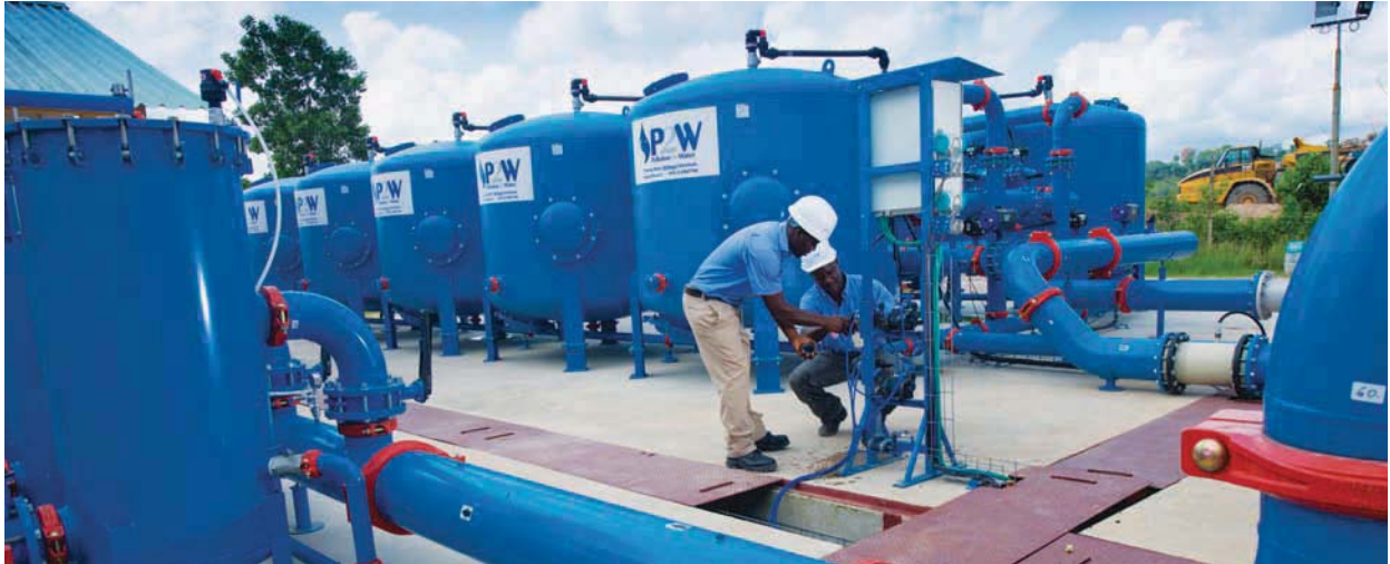
A new water treatment plant is in place at Iduapriem, in Ghana. It uses reverse osmosis to convert used process water from the plant into safe water which is discharged back into the river system near the mine. The process primarily removes the arsenic from the water
