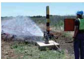
Pump testing a new borehole in the Vaal River area to determine the volume of water that can be pumped on a daily basis
