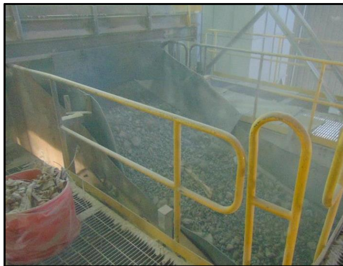
Figure 14-5 – Crushing Plant Screen (Debris Collection and Ambient Dust Visible)
