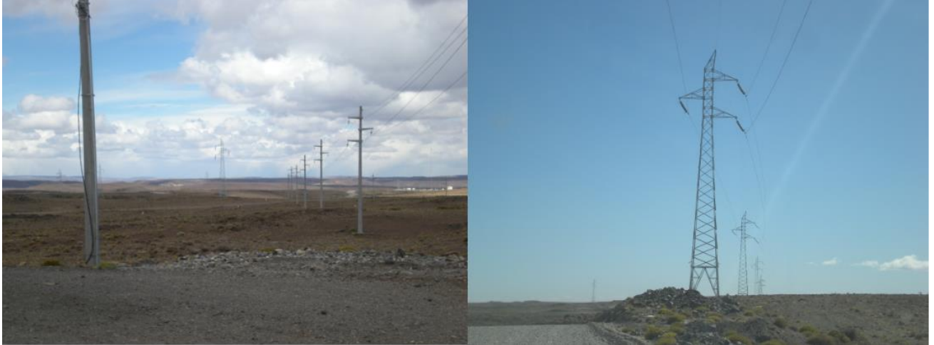
Figure 15-3 – Response of electrical distribution towers to high winds
