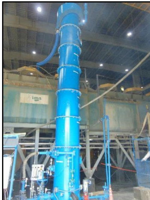
Figure 14-9 – Eriez Column Flotation Cell Installation
